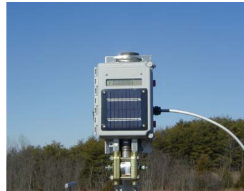
Chart Replacement with 1-Watt Solar Panel
